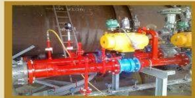
GAS Metering Skid
